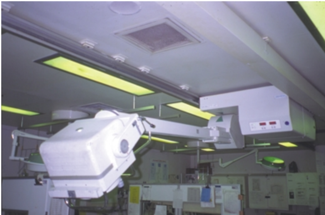
Figure 4.4 Example of a ceiling-mounted X-ray unit for use in trauma imaging centres and a multi-bay environment. Image supplied by the Royal London Hospital.
